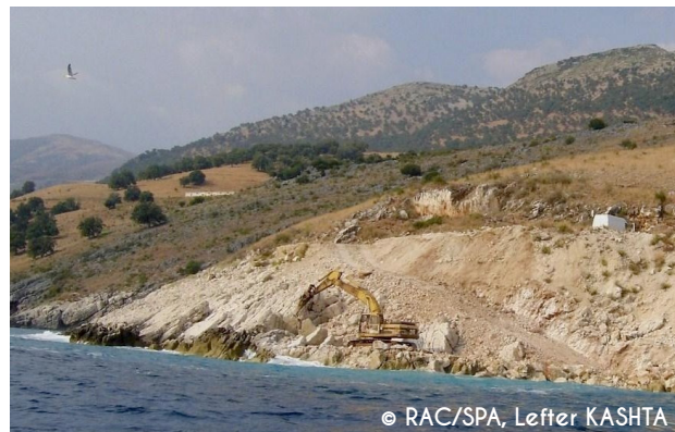
Figure 33. Illegal construction in Porto Palermo coast
